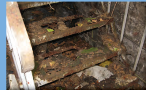
Steel steps after 30 years
